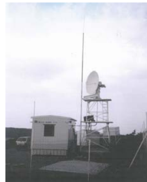
Shelter mounted radar for weather modification project
